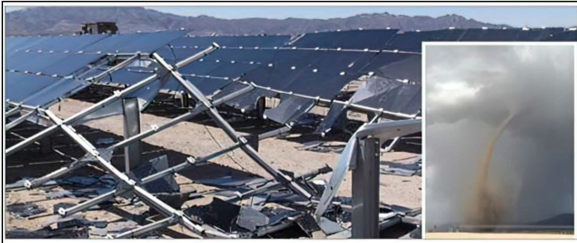
Tornado damage to Desert Sunlight facility in 2015
